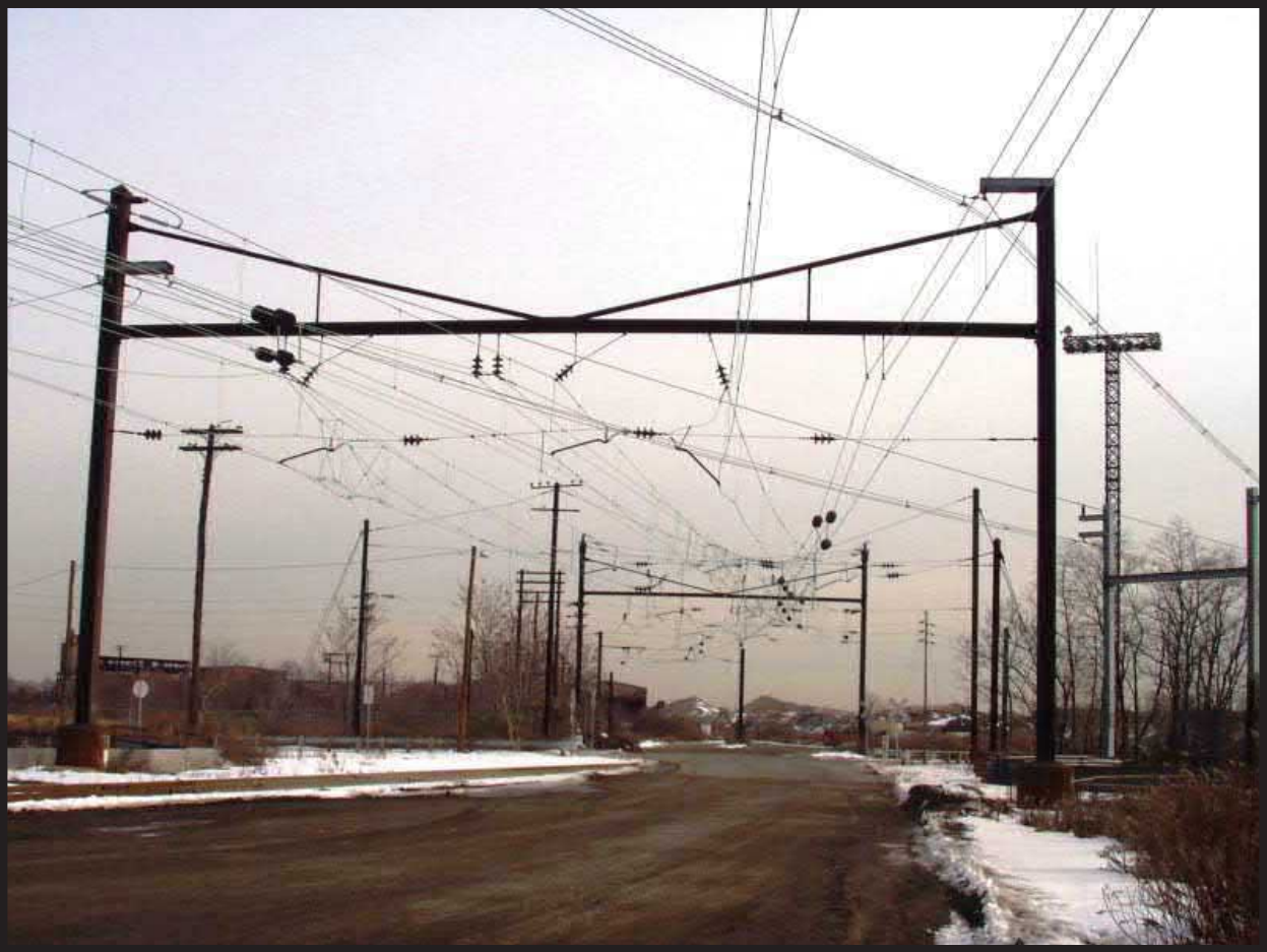
Photograph 5.37. Catenary structure at the South Amboy ferry terminal (Photographer: Ian Burrow, 2002) [HRI Neg. #02081/D1:02].
