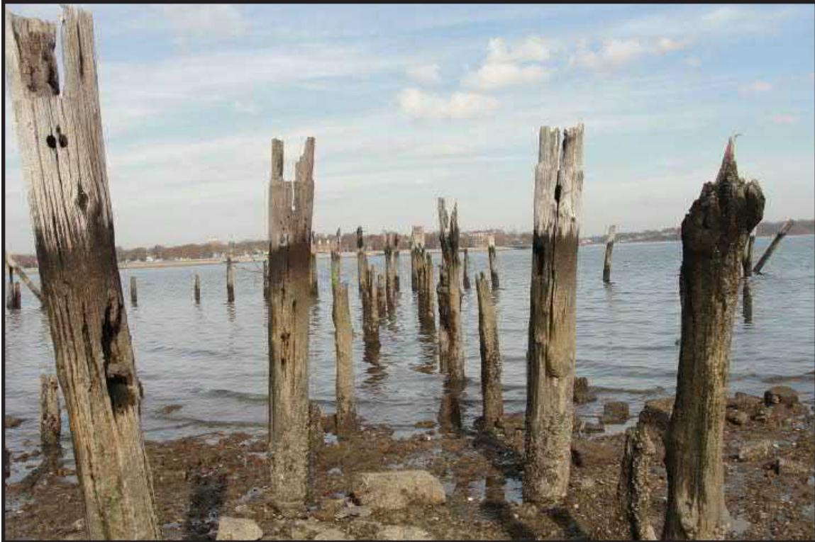
Photograph 7.5. View looking northeast toward Perth Amboy showing the timber supports for the pier which led to the c.1912 barge or “tie-up” racks built by the Pennsylvania Railroad to moor barges awaiting loading from the McMyler coal dumpers installed on the Lehigh pier to the south. The posts at right and left in the middle distance remain from the barge racks themselves (Photographer: Ian Burrow, October 2012) [HRI Neg. #11027/D5:DSC03634].
