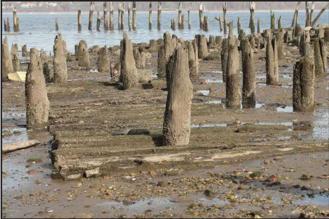
Photograph 7.3. View looking northeast showing the complex horizontal and vertical timbering in the area northwest of the barge rack pier. These support structures lie in the core area of the Camden and Amboy passenger terminal later used by the Pennsylvania Railroad, which also attached freight facilities to the southeast. Some of the timbers are probably of the pre-1871 Camden and Amboy Railroad era (Photographer: Ian Burrow, October 2012) [HRI Neg. #11027/D5:DSC03640].
