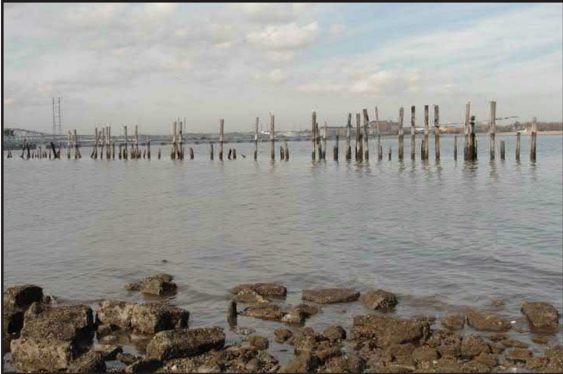
Photograph 7.2. View looking north showing the northern half of the c.1912 barge racks (Photographer: Ian Burrow, October 2012) [HRI Neg. #11027/D5:DSC03630].
