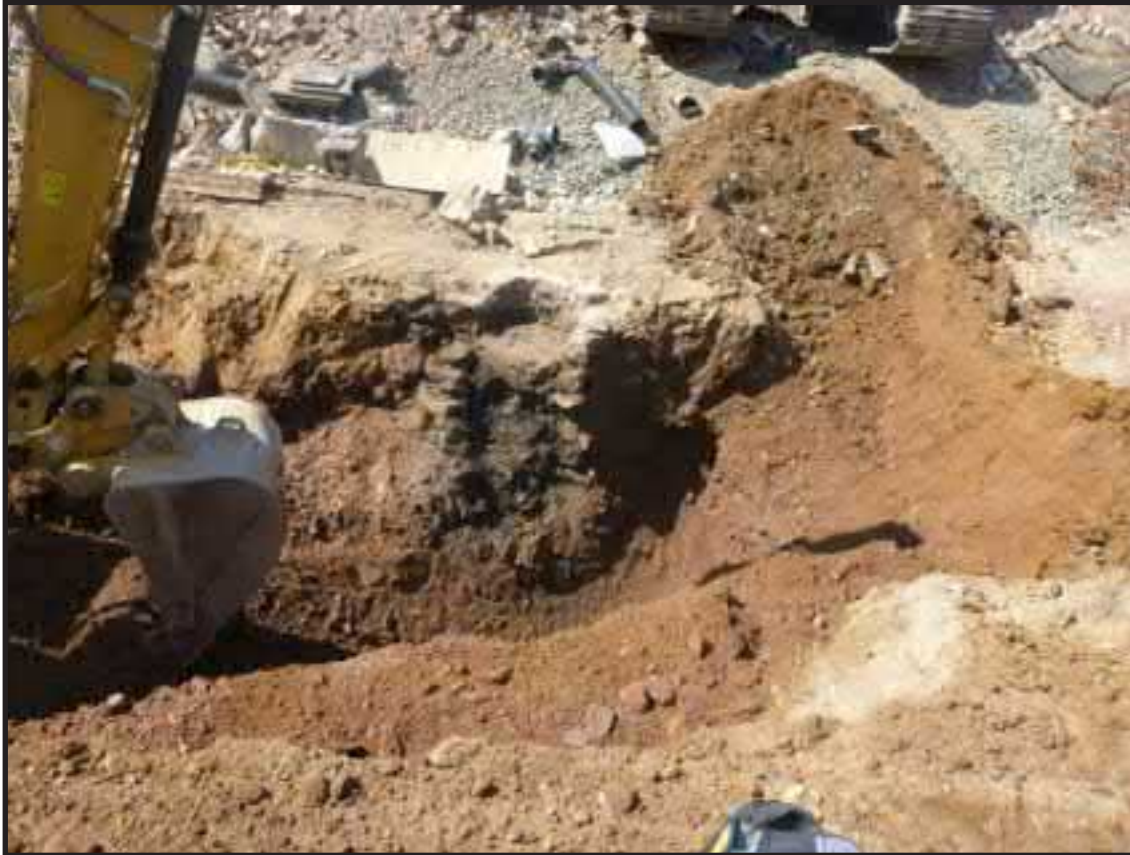
Photograph 4.17. View looking southwest showing a stone-lined well [138, 139] in profile during excavation. This feature was originally built as a well for an early 19th-century dwelling at 71 Halsey Street. The clay drain pipe that connected it to the nearby cistern [125, 126] suggests it was repurposed as a drain; scales in feet (Photographer: Joshua Butchko, June 2017) [HRI Neg.# 17033/D7:051].
