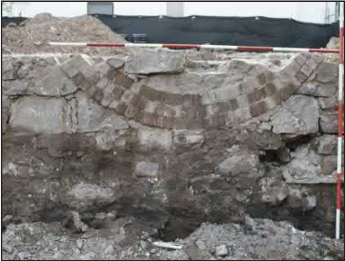
Photograph 4.6. View facing north showing an inverted brick vault under a basement window lintel in the north foundation wall [1163] of the Halsey Street Methodist Episcopal Church; scales in feet (Photographer: Michael Brown, July 2017) [HRI Neg.# 17033/D6:2051].
