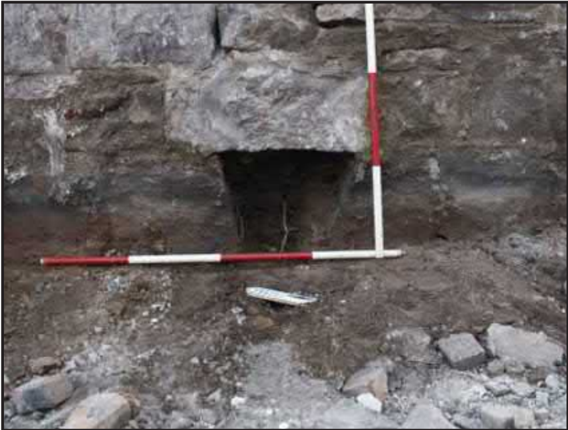
Photograph 4.8. View facing north showing a void, probably a ventilation channel, built into the north foundation wall [1163] of the Halsey Street Methodist Episcopal Church; scales in feet (Photographer: Michael Brown, July 2017) [HRI Neg.# 17033/D6:2056].
