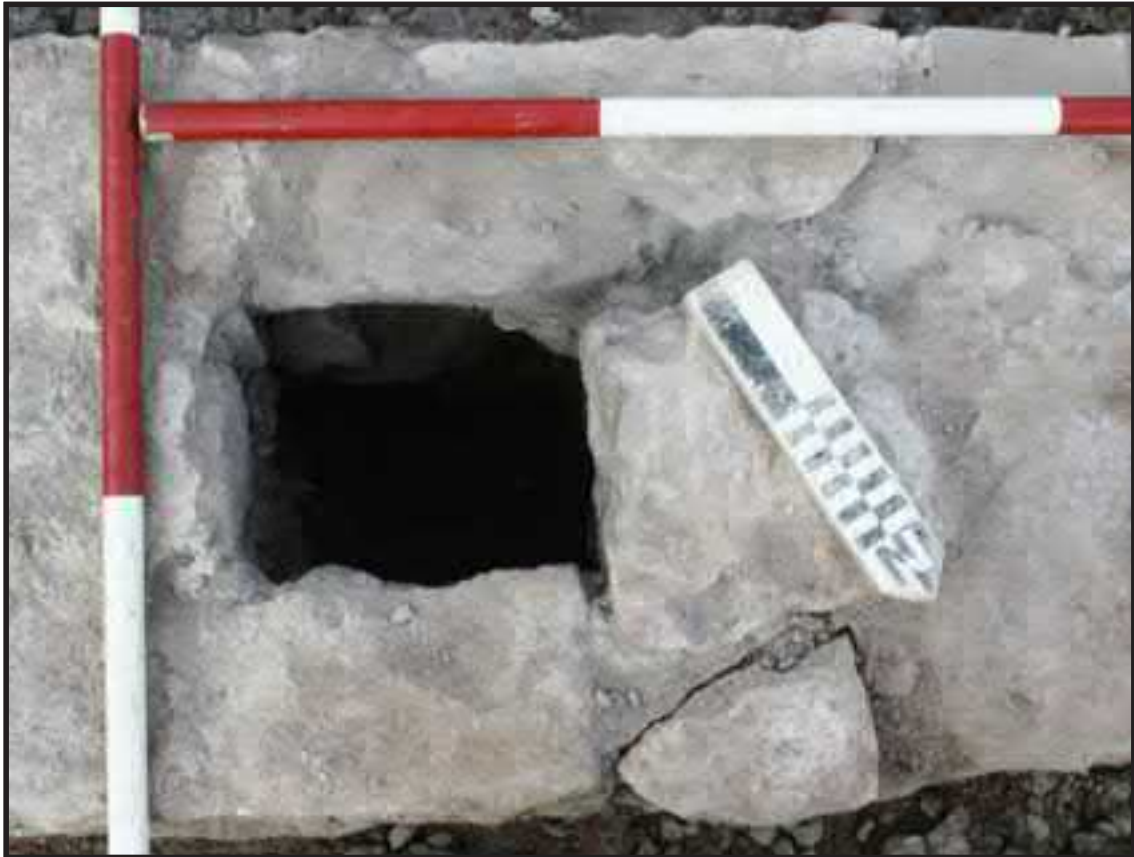
Photograph 4.9. Plan view showing void (ventilation channel) within the north foundation wall [1163] of the Halsey Street Methodist Episcopal Church; scales in feet (Photographer: Michael Brown, July 2017) [HRI Neg.# 17033/D6:2082].
