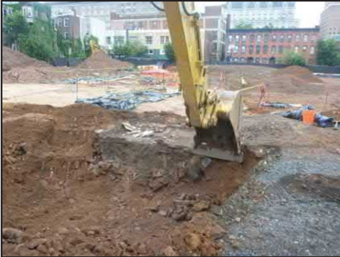
Photograph 3.16. View facing southeast showing the excavation in progress of the privy in the rear yard of 54 and 56 New Street. Excavation around the north side of the privy shaft allowed for the disassembly of its masonry walls and the exposure of its contents in cross-section (Photographer: Josh Butchko, July 2017) [HRI Neg.# 17033/D10:004].
