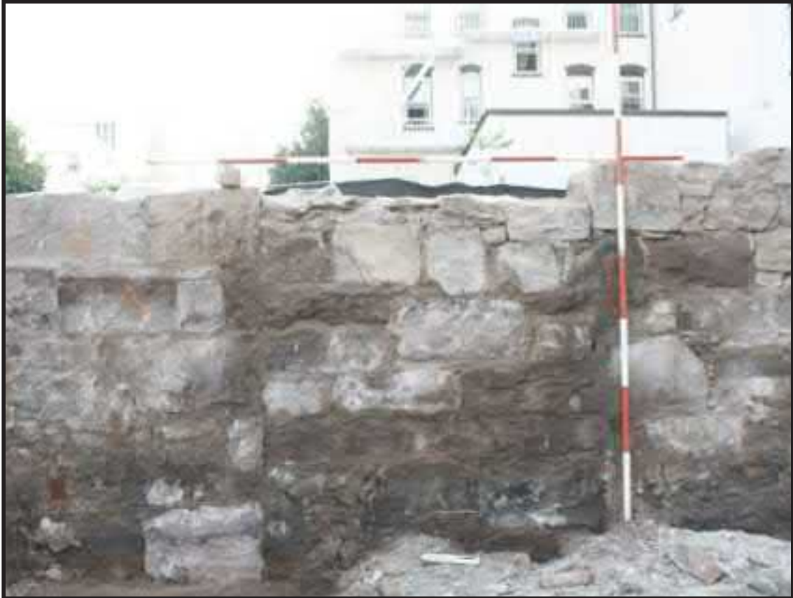
Photograph 4.7. View facing north showing a blocked basement doorway in the north foundation wall [1163] of the Halsey Street Methodist Episcopal Church; scales in feet (Photographer: Michael Brown, July 2017) [HRI Neg.# 17033/D6:2038].
