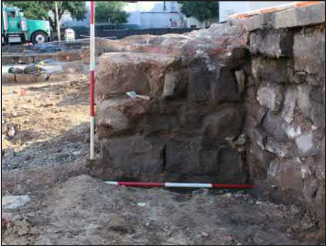
Photograph 4.11. View facing east toward New Street showing the relationship between the brownstone chimney base [1039] and the rear wall [1022] of the Halsey Street Methodist Episcopal Church. Note that the base is not keyed into the church wall; scales in feet (Photographer: Michael Brown, June 2017) [HRI Neg.# 17033/D13:3731].
