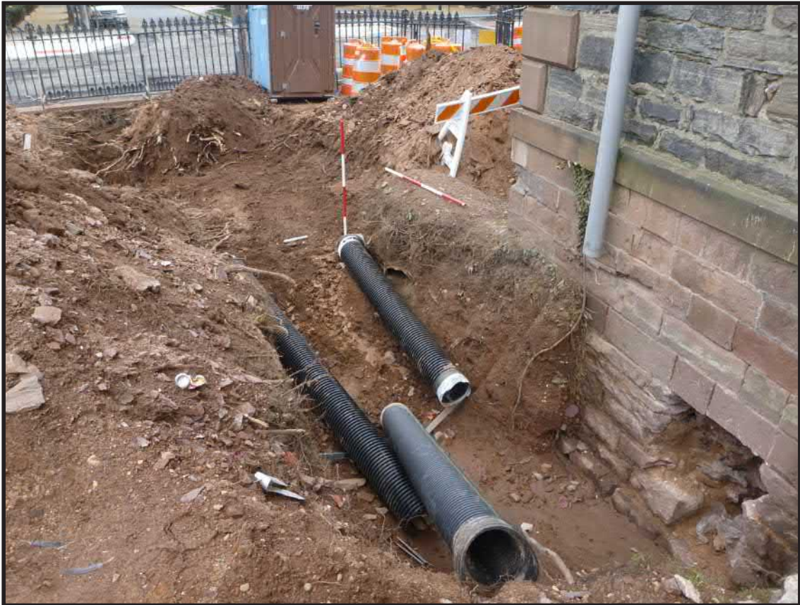
Photograph 4.9. View looking east showing Trench 8 fully excavated and awaiting installation of utilities. Scales in feet (Photographer: Joshua Butchko, October 2015) [HRI Neg. #15004/D4:059].
