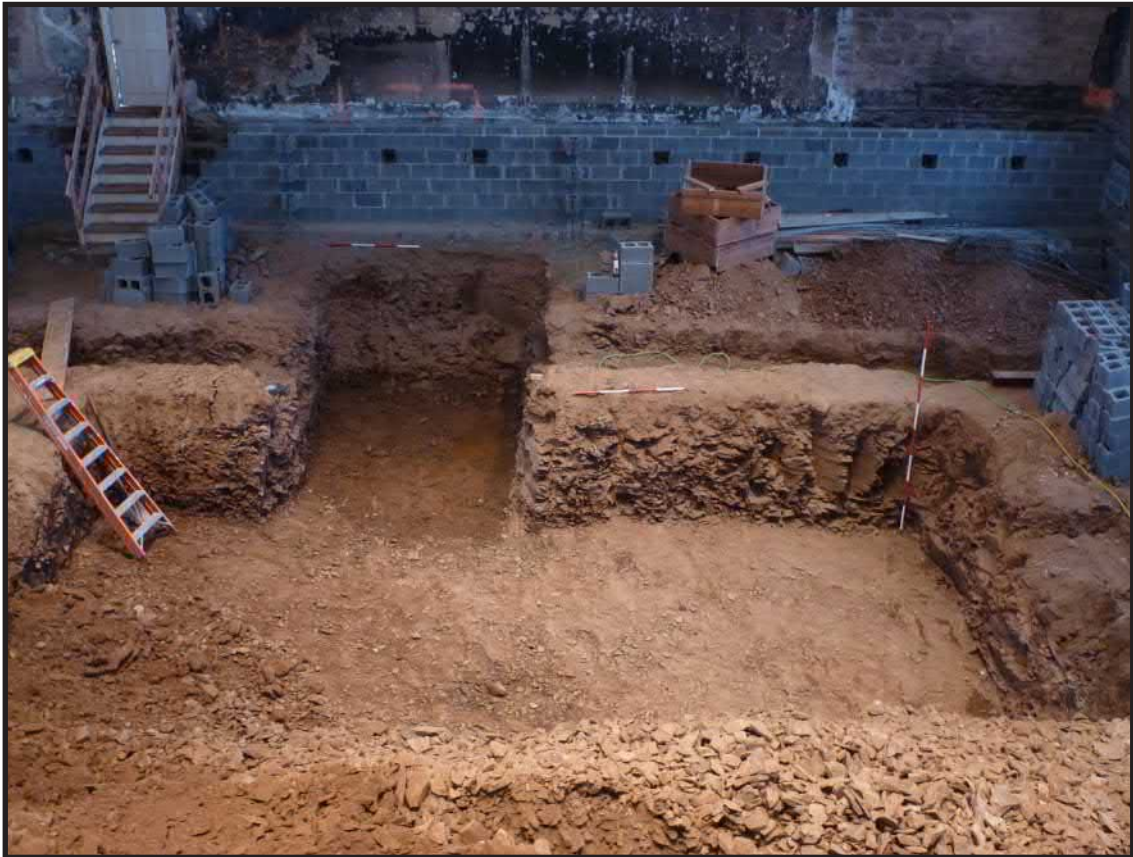
Photograph 3.28. View looking west showing the fully excavated Basement Excavation Area at the western end of the auditorium. Note the cinderblock foundation has been installed to reinforce the interior face of the church’s western foundation. Scales in feet (Photographer: Joshua Butchko, March 2015) [HRI Neg. #15001/D6:052].
