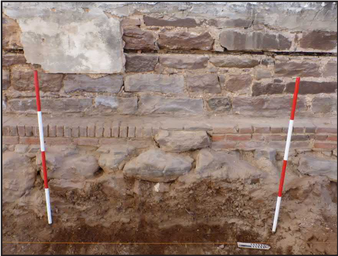
Photograph 3.16. View looking west showing part of the church’s west wall and foundation. The top of the two to three courses of brick masonry represents the level of the first floor in the auditorium. The wood nailer above has a section wall plaster still attached. The stone masonry beneath the bricks is conjectured to be part of the foundation of the original church built in 1767 re-used in the present church of 1811-12. Scales in feet and tenths of feet (Photographer: Joshua Butchko, February 2015) [HRI Neg. #15001/D3:030].
