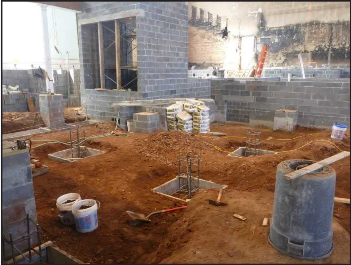
Photograph 3.31. View looking southwest showing the progress of interior construction following completion of most of the excavation monitoring (Photographer: Joshua Butchko, March 2015) [HRI Neg. #15001/D8:264].
