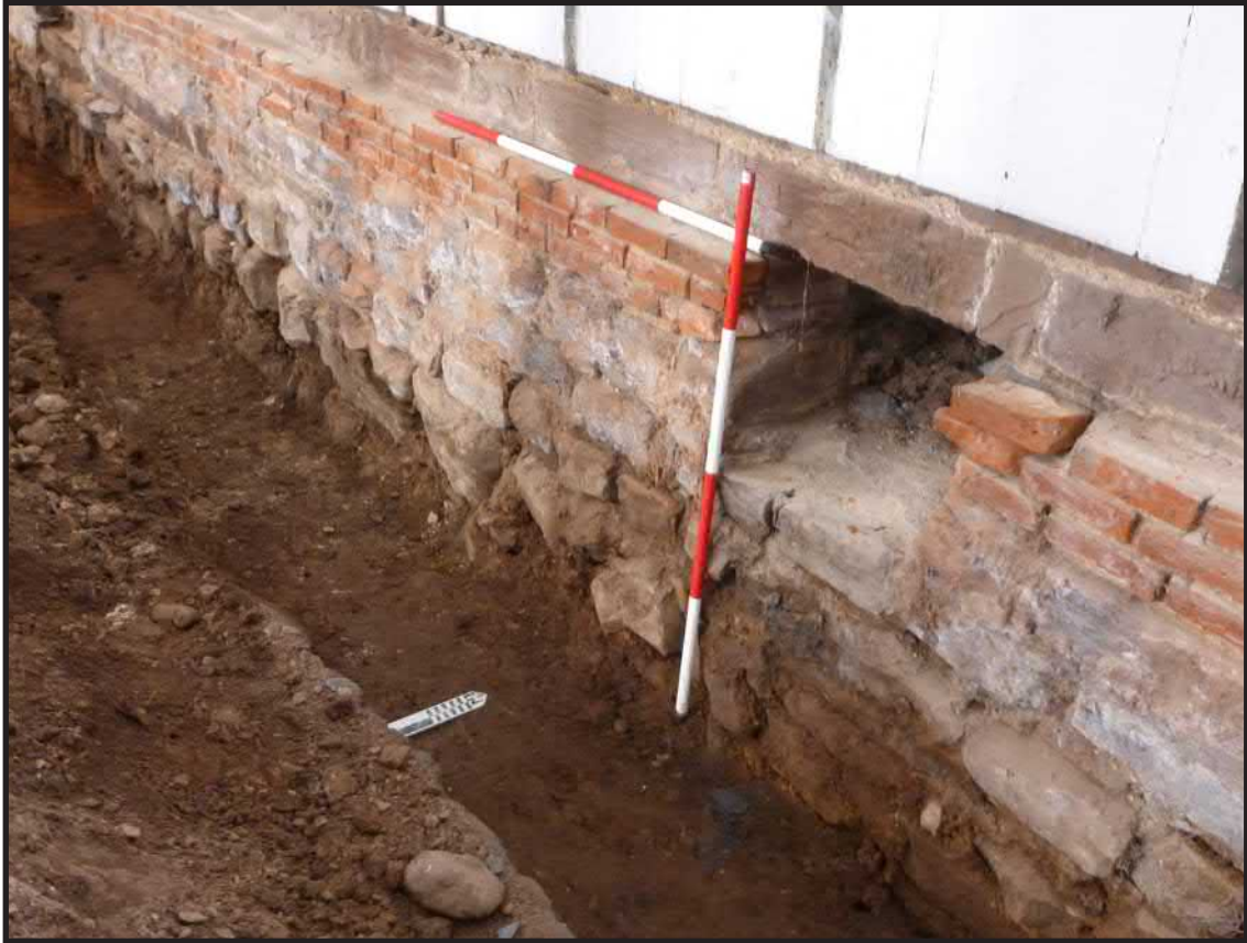
Photograph 3.10. View looking northwest midway along Trench 1. In the floor of the trench to the left of the north arrow/small scale rod is a concentration of mortar, plaster and rubble cut into by the foundation for the church’s north wall. This material is thought to be the fill of a robber trench reflecting the removal of the foundation for the northeast corner of the original church of 1767 or of a north-south wall that extended north beyond the footprint of the original church. The top surface of the three courses of brick masonry represents the first-floor level of the auditorium. The rectangular recess in the foundation to the right of the vertical scale pole is a joist pocket for one of the principal members of the first-floor framing. Scales in feet and tenths of feet (Photographer: Joshua Butchko, February 2015) [HRI Neg. #15001/D2:237].
