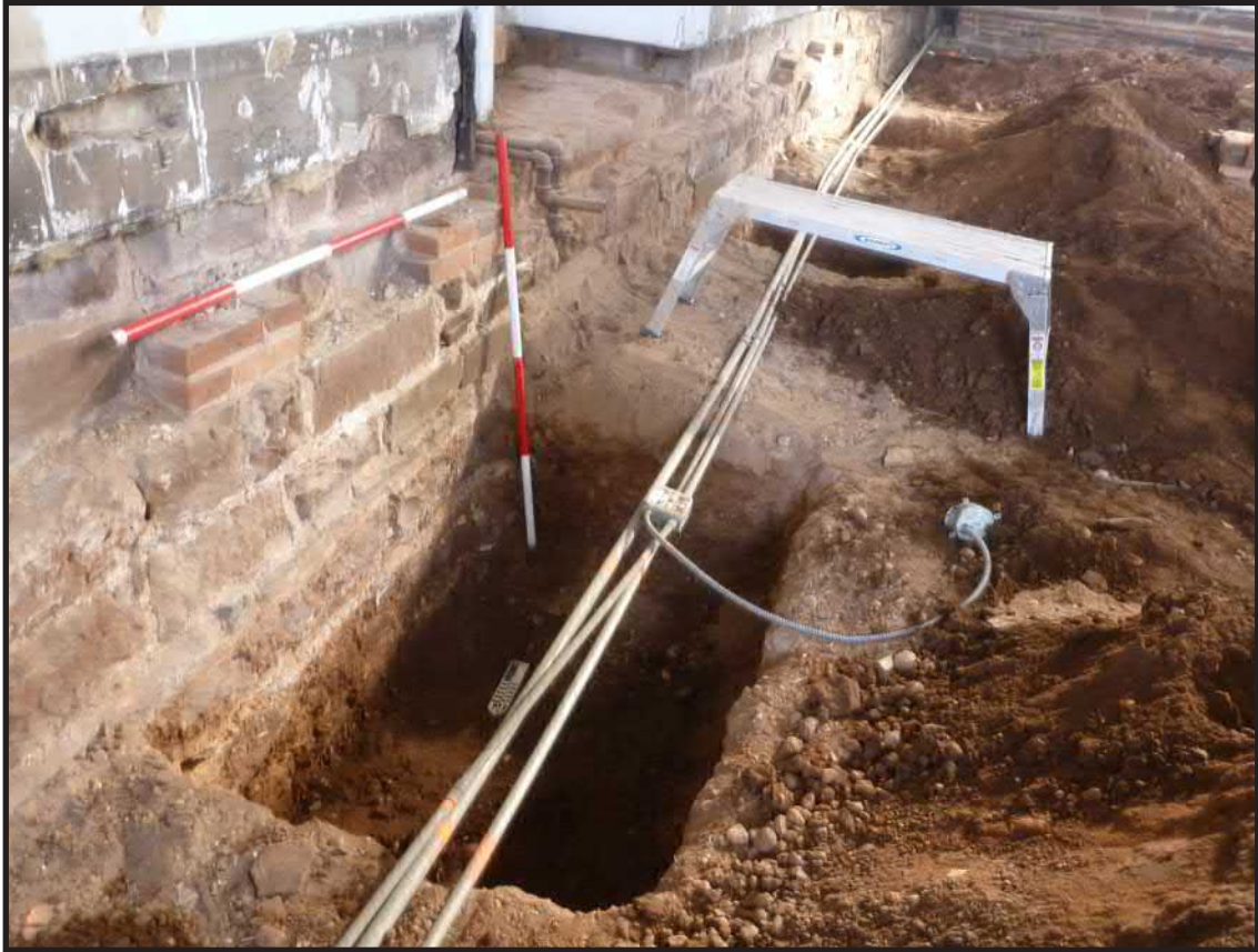
Photograph 3.25. View looking south southeast along the face of east wall of the auditorium showing the excavations for Pier Footings 9, 14 and 17. Scales in feet (Photographer: Joshua Butchko, February 2015) [HRI Neg. #15001/D3:096].
