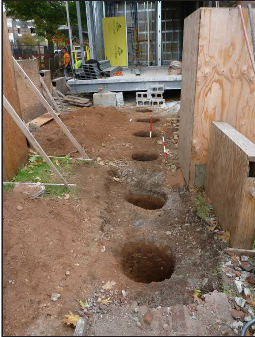
Photograph 4.10. View looking north showing Sonotube Pits 1-6 which were excavated for the footings of an ADA-compliant ramp providing access into the rear of the church. Scales in feet (Photographer: Joshua Butchko, October 2015) [HRI Neg. #15004/D4:073].
