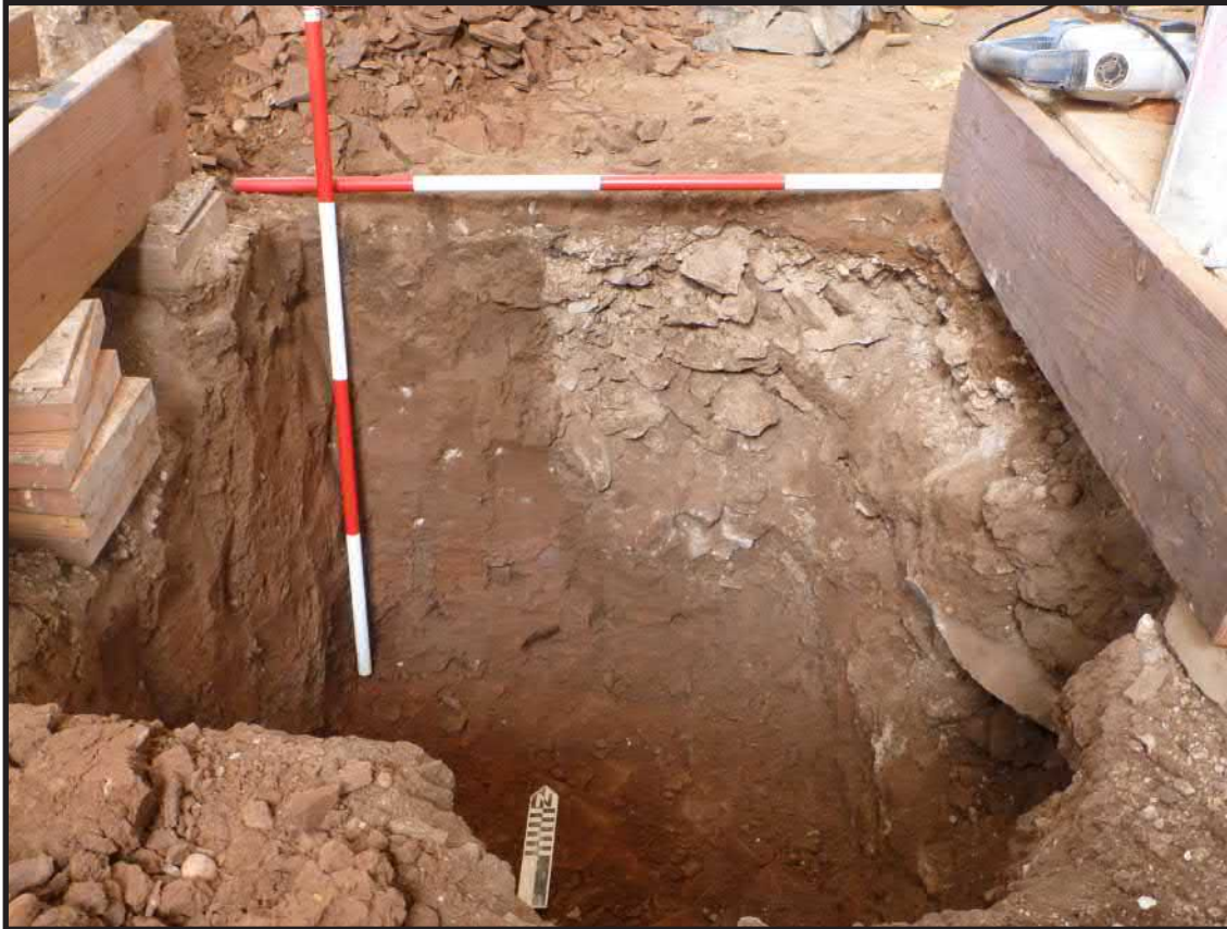
Photograph 3.26. View looking north showing the north profile of the excavation pit for Pier Footing 15. To the right of the vertical scale pole is the cut and rubble fill of the robber trench resulting from the removal of the foundation for the east wall of the original church built in 1767. Scales in feet and tenths of feet (Photographer: Joshua Butchko, February 2015) [HRI Neg. #15001/D3:080].
