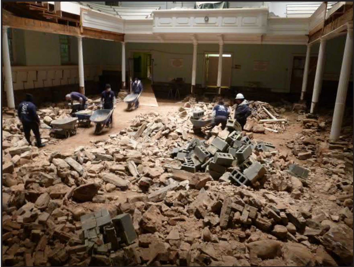
Photograph 3.2. View looking east-northeast showing the contractor removing the demolished first-floor foundations. Note the stone footings underpinning the wooden columns supporting the second-floor balcony (Photographer: Joshua Butchko, January 2015) [HRI Neg. #15001/D1:060].
