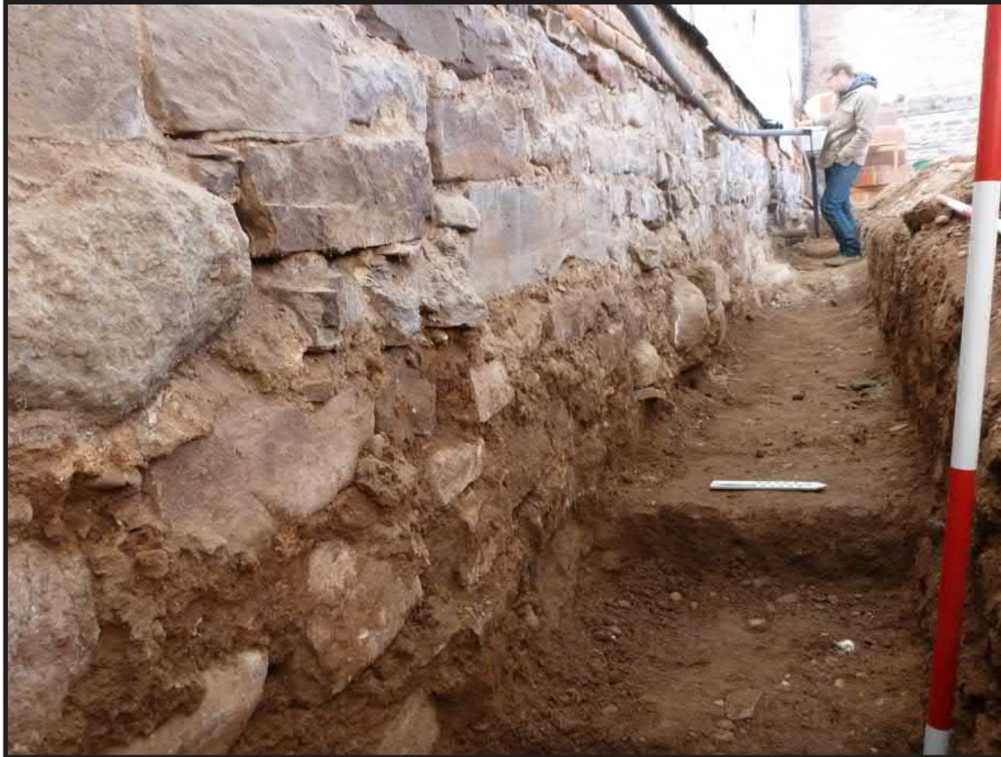
Photograph 3.11. View looking west showing Trench 2 fully excavated. At left is the stone masonry of the church's south wall foundation capped with three courses of brick on top of which the first floor of the auditorium was set. Scales in feet and tenths of feet (Photographer: Joshua Butchko, February 2015) [HRI Neg. #15001/D3:108].
