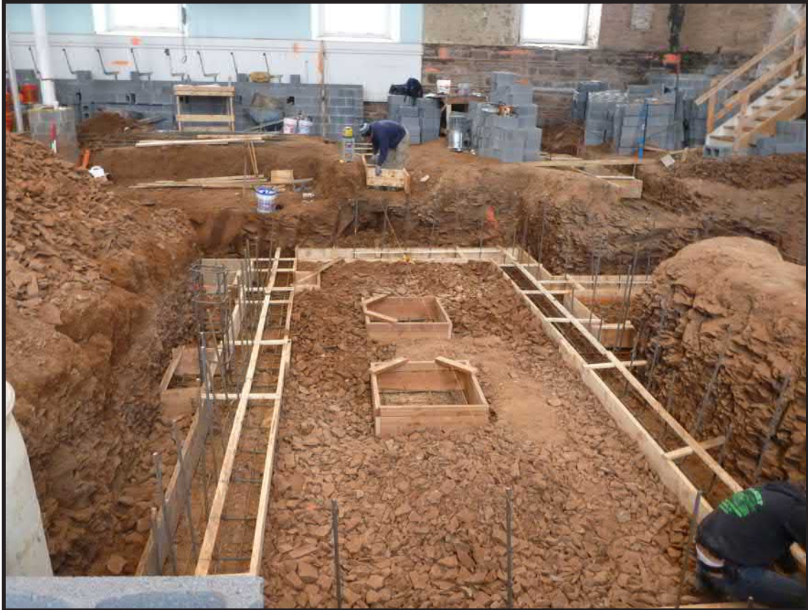
Photograph 3.29. View looking south showing the Basement Excavation Area with the installation of new footings in progress (Photographer: Joshua Butchko, March 2015) [HRI Neg. #15001/D6:169].
