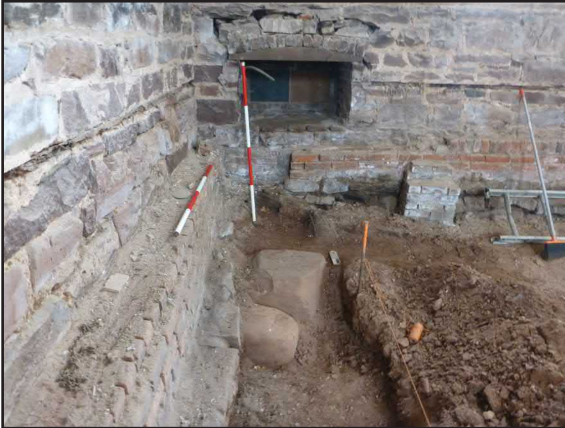
Photograph 3.15. View looking north showing the northern end of Trench 3 in the northwest corner of the auditorium. Note the four courses of brick masonry on top of the western stone foundation at left and three courses on the northern foundation at right, on top of which the first-floor framing for the dais was originally set (it was later raised to a higher elevation). A wooden nailer for lath and plaster wall covering is visible running horizontally in the west wall at left. The brick-arched opening with cast-iron lintel in the north wall in the center of the view is a former window opening inserted in the later 19th century to provide light for a stair giving access to the crawlspace. The large blocks of stone in the foreground are considered to be remnants of the northwest corner of the original church built in 1767. Scales in feet and tenths of feet (Photographer: Joshua Butchko, January 2015) [HRI Neg. #15001/D2:246].
