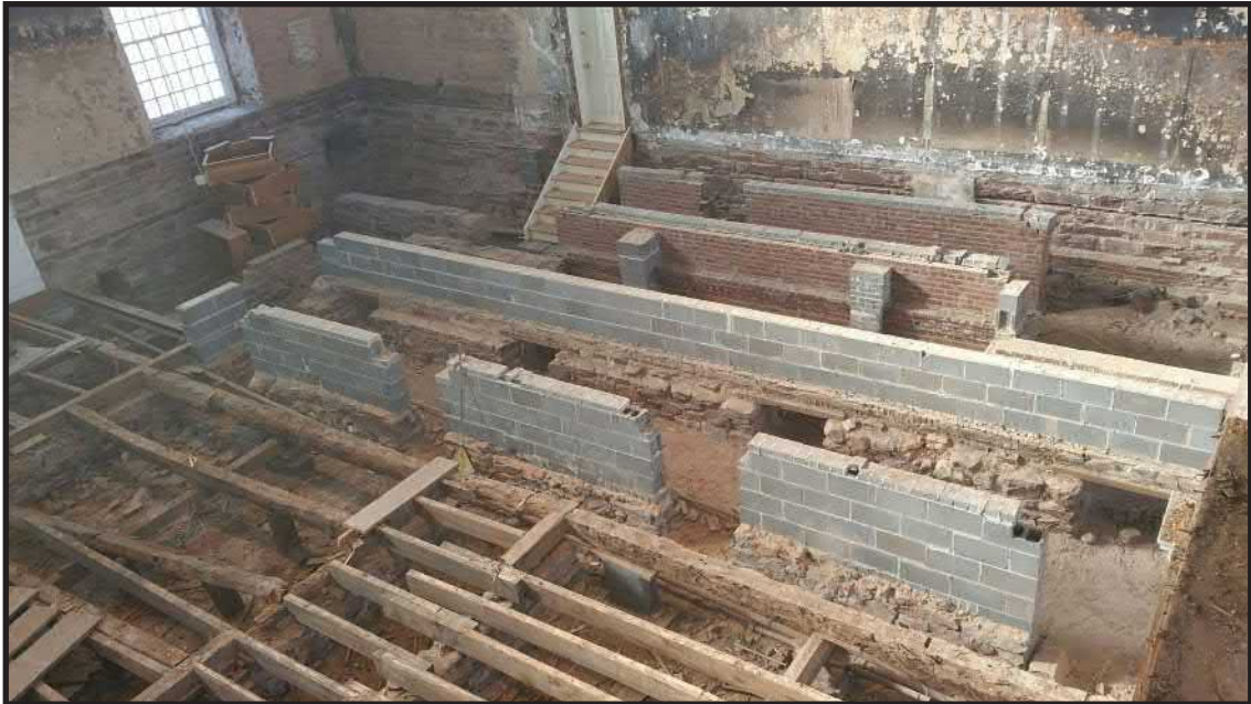
Photograph 3.1. View looking southwest showing exposed floor joists and stone, brick and cinder-block foundations supporting the first floor of the church auditorium and sanctuary. The cinderblock and brick foundations supported an elevated dais in the sanctuary at the western end of the building (Photographer: E-Tomic Construction Services, January 2015).
