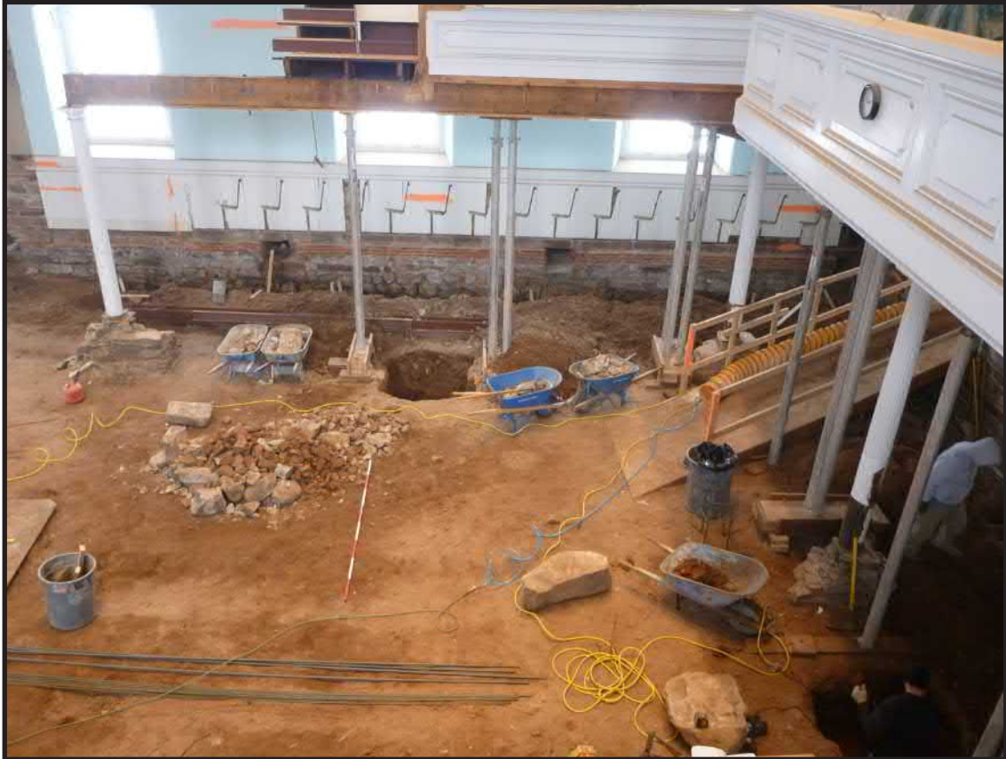
Photograph 3.21. View facing north showing the church interior at the start of pier footing excavations. The deep excavation between the temporary props holding up the balcony was dug to allow installation of a temporarily removed wood column on a new concrete and cinderblock footing (Pier Footing 1). Scale in feet (Photographer: Joshua Butchko, February 2015) [HRI Neg. #15001/D3:179].
