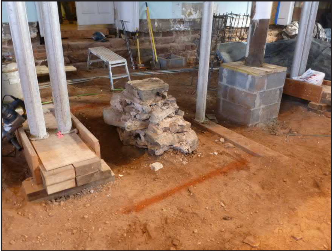
Photograph 3.23. View looking southeast showing the original mortared stone footing for the column that supported the second-floor balcony on the north side of the main aisle (the column has been temporarily removed to allow for replacement of the footing) (Pier Footing 8). The footing for the companion column on the south side of the main aisle has been replaced (Pier Footing 12) and the entire area has by this time been excavated down to the base of the new and old pier footings (Photographer: Joshua Butchko, February 2015) [HRI Neg. #15001/D5:194].
