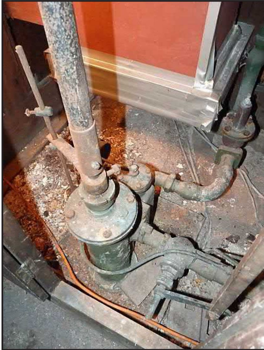
Photograph 3.6. A Water Engine Installed in 1901 and Still Used to Power the Pipe Organ at St Michael's & All Angels Church in Averham, Nottinghamshire, England. Source: Self 2017.
