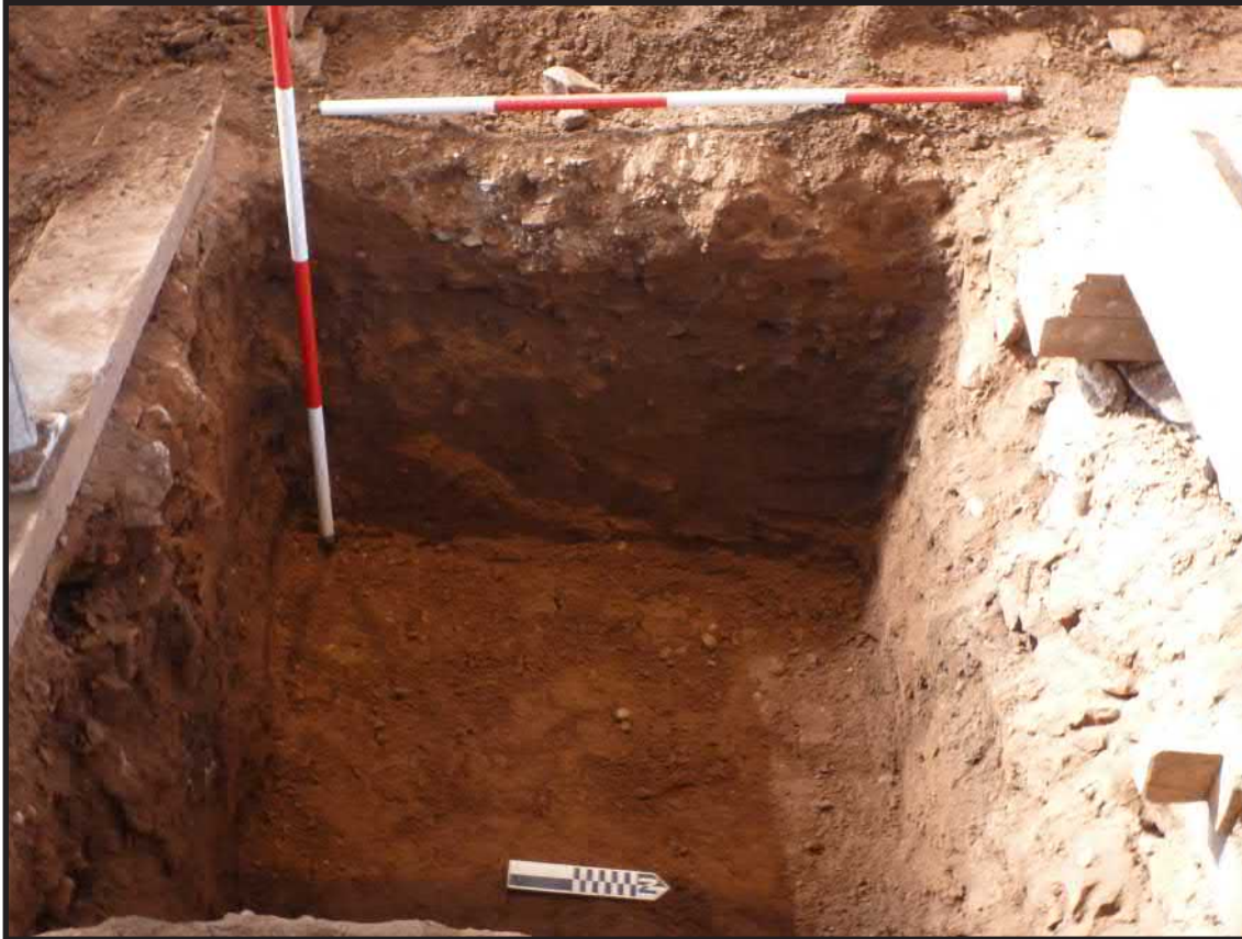
Photograph 3.24. View looking west showing the completed excavation for Pier Footing 8 which facilitated the removal and replacement of the mortared stone footing for the wood column that supported the second-floor balcony on the north side of the main aisle. Scales in feet and tenths of feet (Photographer: Joshua Butchko, February 2015) [HRI Neg. #15001/D5:215].
