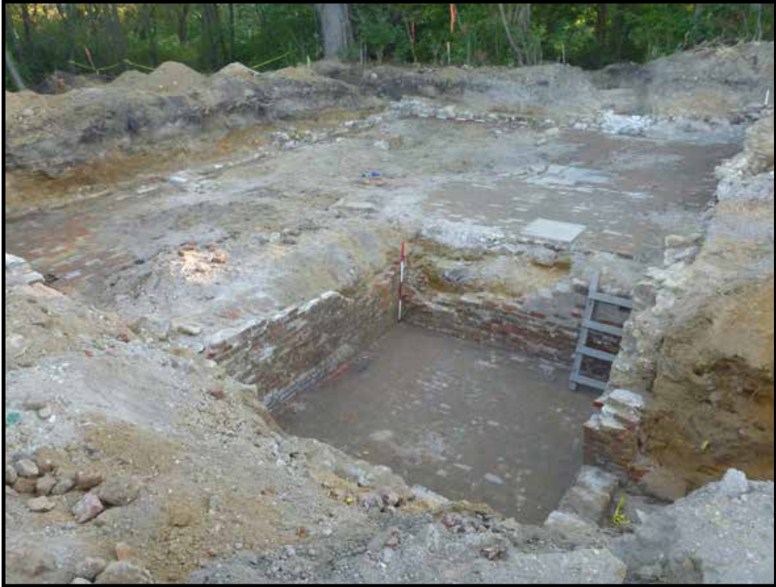
Photograph 3.17. View looking southwest showing final view of the Borton/Ballinger Farm House basement floor plan (Photographer: Joshua Butchko, September 2016) [HRI Neg. #16034/D3:365].
