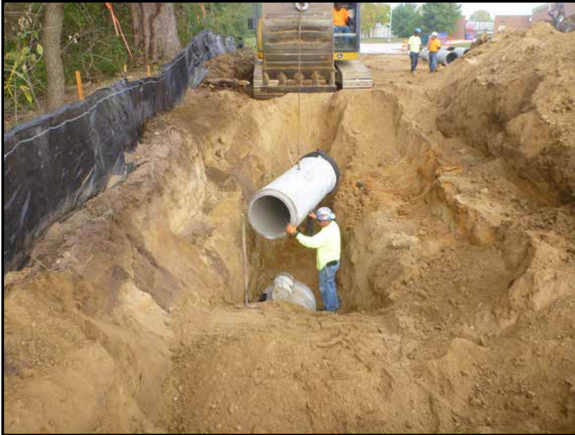
Photograph 3.27. View looking northwest showing installation of new pipeline along west edge of proposed road across Borton/Ballinger Farm House Site observed during archaeological monitoring program of new construction (Photographer: Andrew Martin, October 2016) [HRI Neg. #16034/D5:010].
