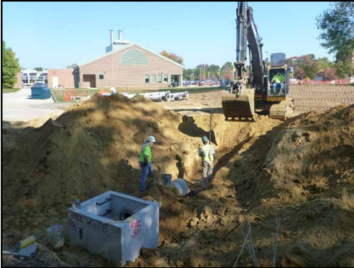
Photograph 3.29. View looking north-northeast showing pipe trench excavation continuing beyond northern limit of project area observed during archaeological monitoring program of new construction (Photographer: Joshua Butchko, October 2016) [HRI Neg. #16034/D6:064].
