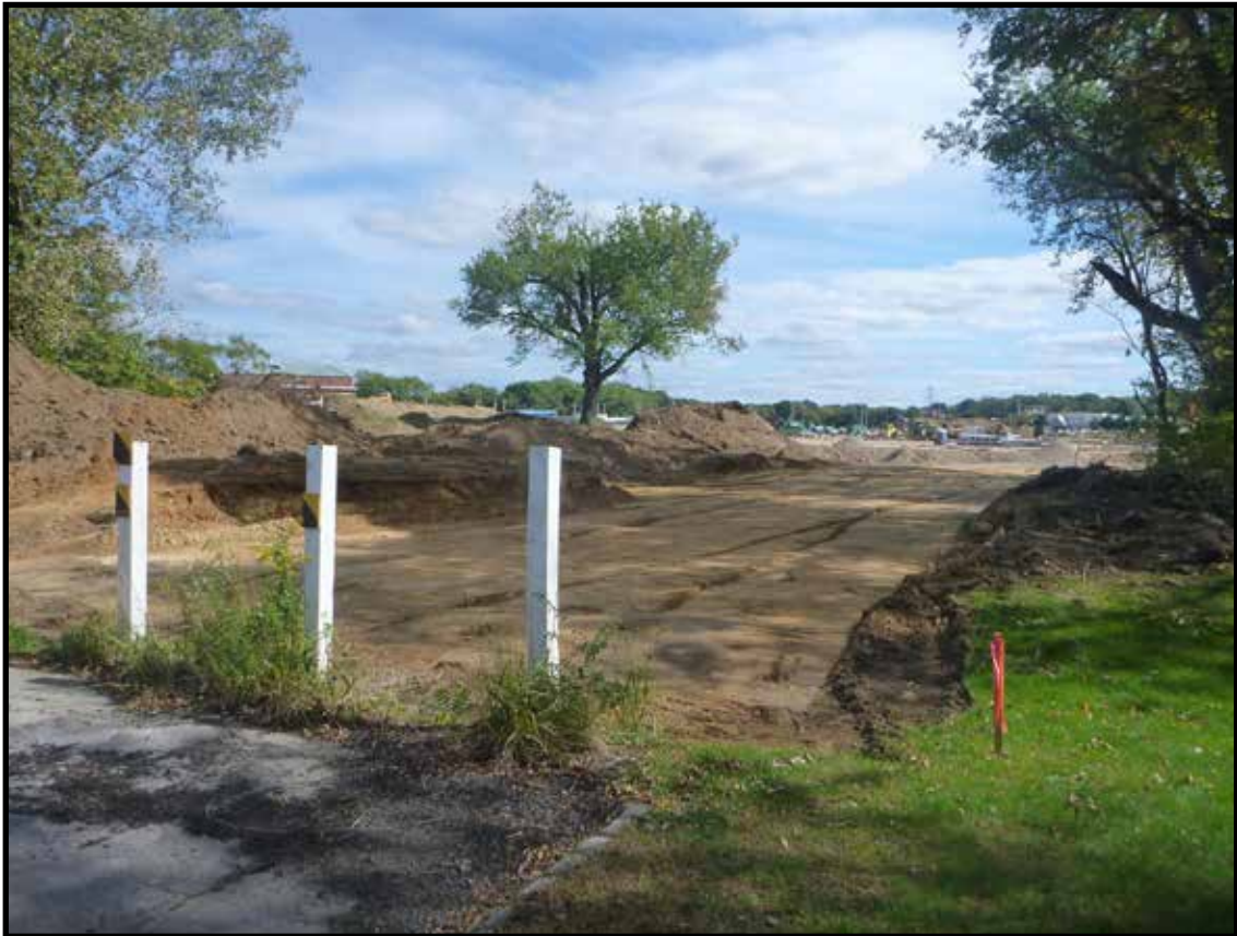
Photograph 3.26. View looking east-southeast showing final grade for proposed road at Borton/Ballinger Farm House Site observed during archaeological monitoring program of new construction (Photographer: Joshua Butchko, October 2016) [HRI Neg. #16034/D4:094].
