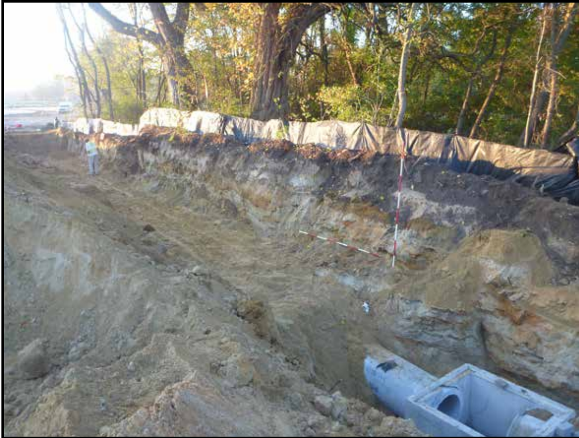
Photograph 3.28. View looking south showing partial west profile of pipe trench excavation observed during archaeological monitoring program of new construction (Photographer: Joshua Butchko, October 2016) [HRI Neg. #16034/D6:035].
