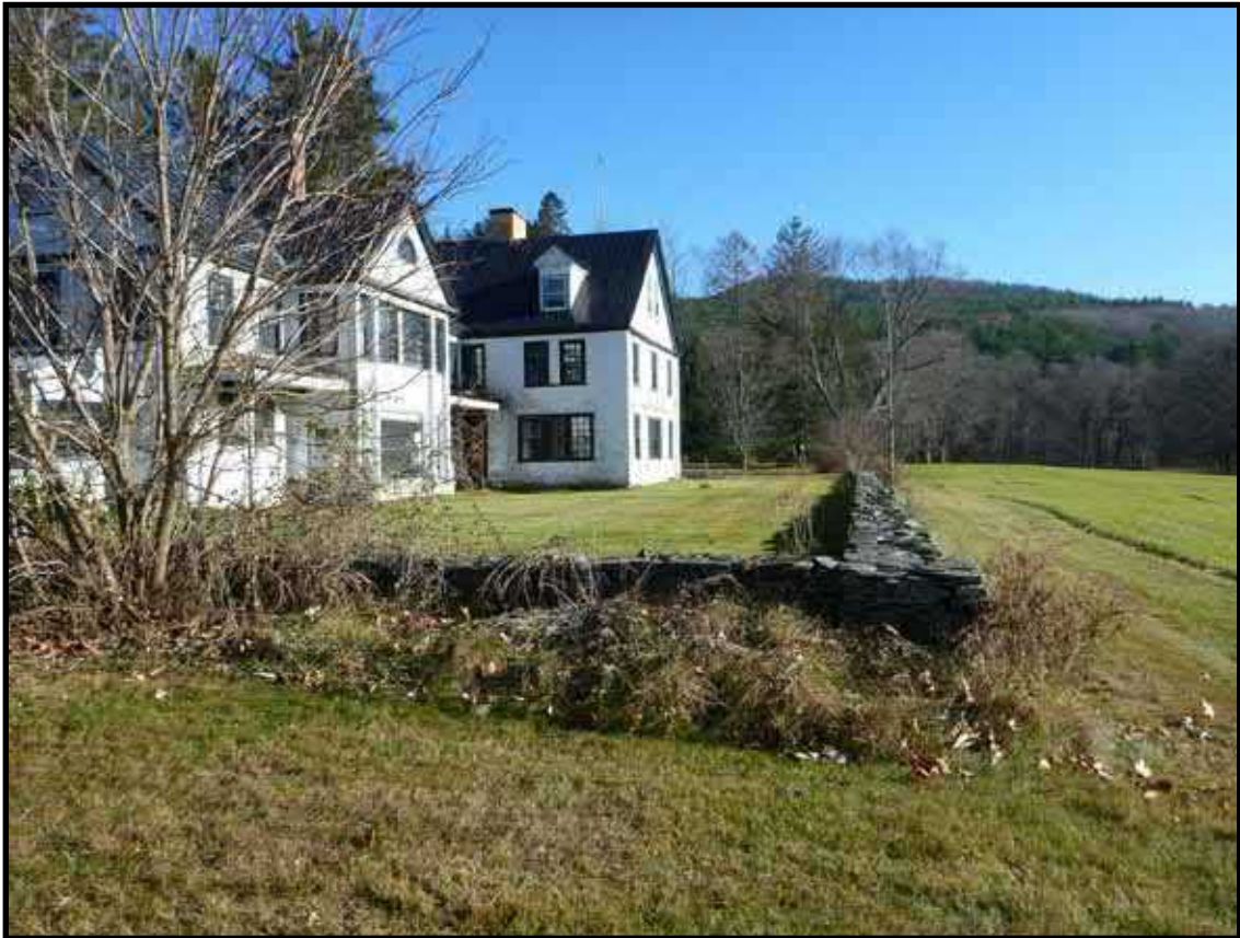
Photograph 6.15. View southeast showing the dry-laid stone retaining wall just west of the casino (photographer: James Lee, November 2016) [HRI Neg.#16048/D2-147].
