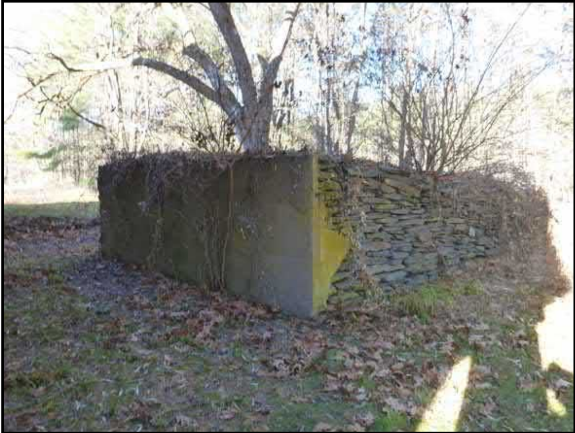
Photograph 6.21. View northeast showing the stone and earthen ramp at the eastern end of the Barn (photographer: James Lee, November 2016) [HRI Neg.#16048/D2-99].
